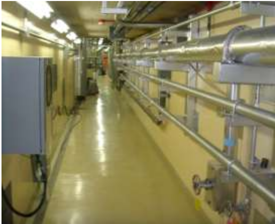
R/B Walkway, Unit 1
